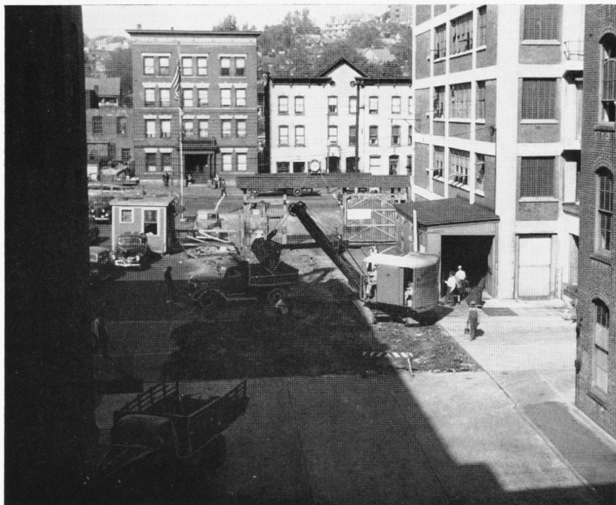
Steam shovel breaking ground for a wider and improved entrance at the Hayden Street Gate. The work is being done by the Turner Construction Company under the supervision of the Administrative Engineering Department. When completed a two-way traffic lane will lead into the factory and a new gate house will supplant the present one.
