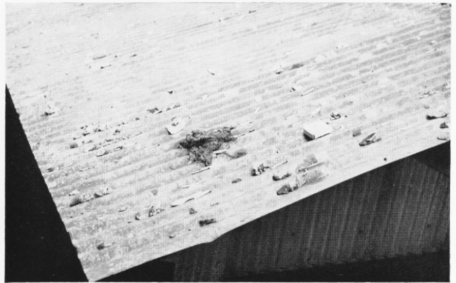
Here's a picture that shows the results of the dangerous habit of tossing cigarettes and matches. Many of them litter this metal roof. Some burned out after landing on the roof which, fortunately, is fireproof. The careless habit is widespread, but that doesn't make it the less dangerous.
